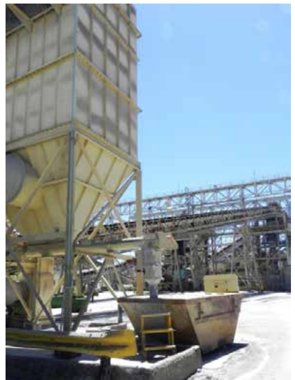
Figure 20: Fine crushing dust collection system
